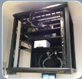
EQUIPMENT RACK AT CENTRAL LOCATION
